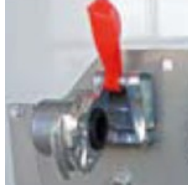
In-correct Application / Hatalı Uygulama
